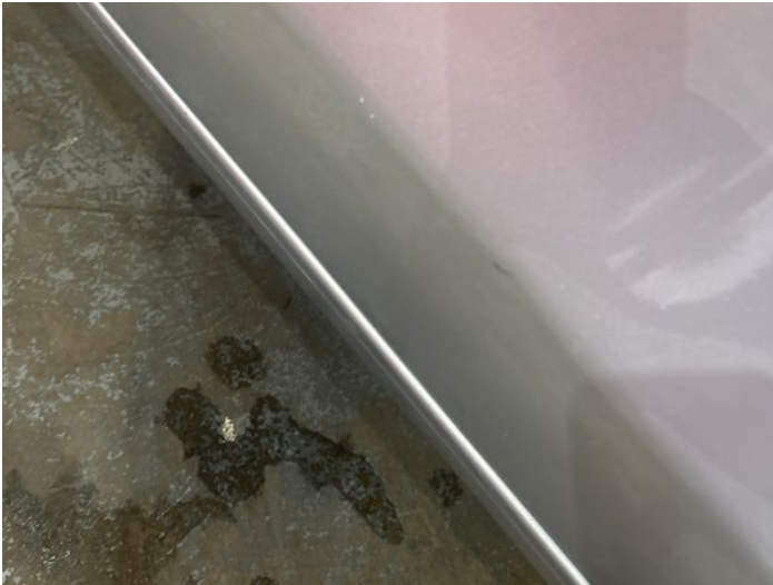
3: Door osf Chipped 1 To 5
