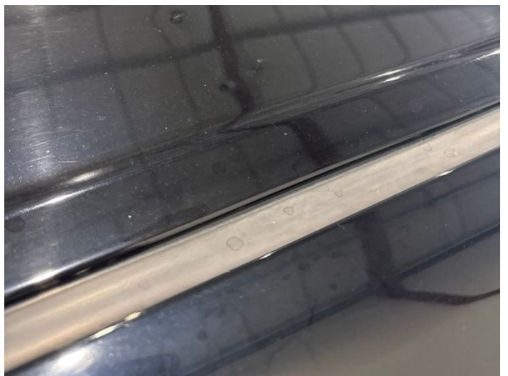
14: Roof Dented Over 30mm
