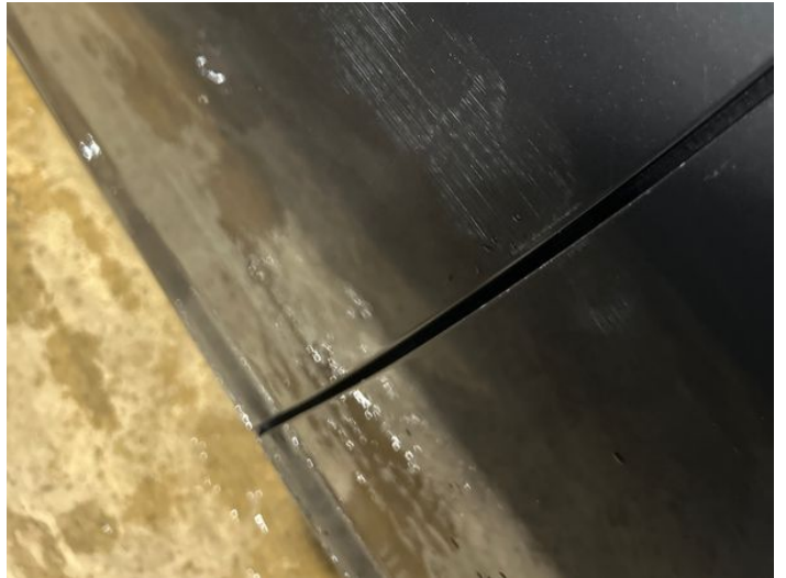
4: Door osr Scratched Over 25mm Thru Paint
