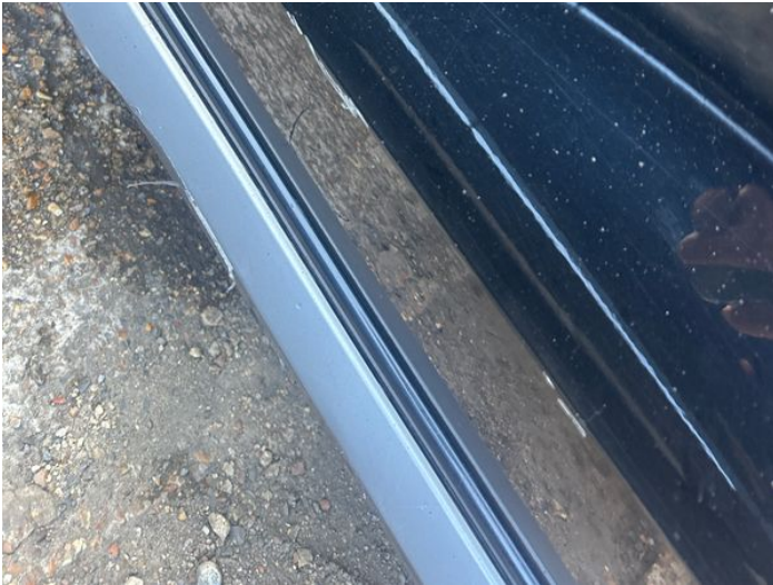
9: Door nsf Scratched Over 25mm Thru Paint
