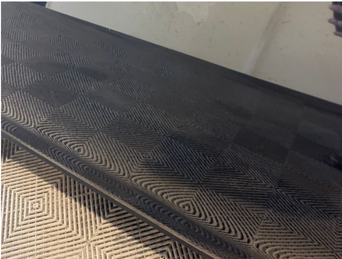
5: Door nsf Poor Previous Repair Paint Flake
