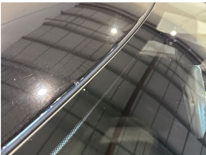
18: Roof Chipped Edge Chip
