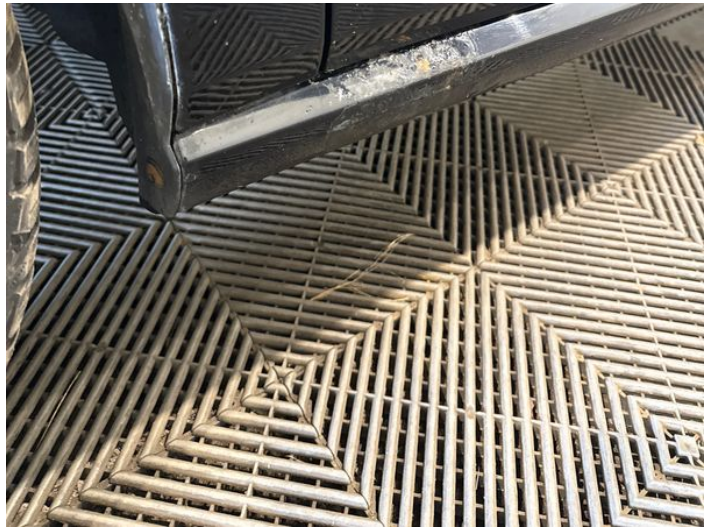
6: Sill ns Rusted Over 5mm
