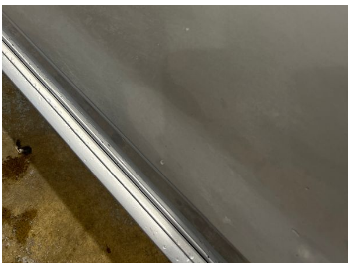
5: Door nsf Chipped 1 To 5
