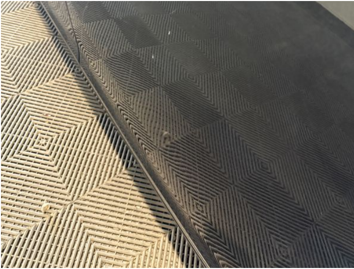
9: Door nsr Poor Previous Repair Rippled UpTo 30%
