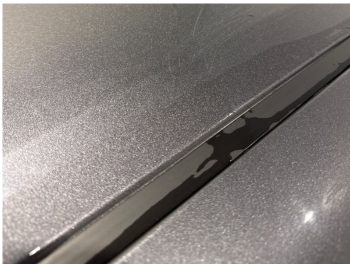
1: Roof Scratched Over 25mm Thru Paint
