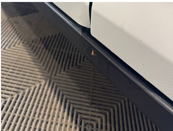
5: Door nsf Dented Between 10mm + 30mm
