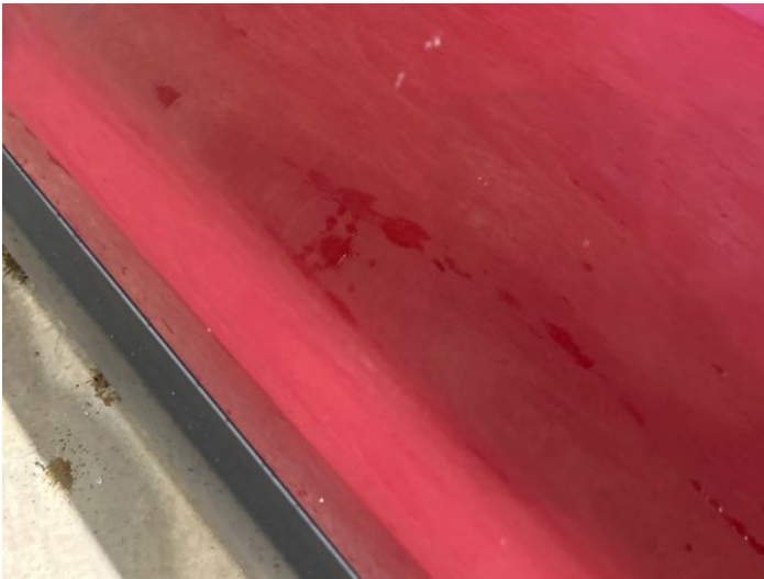
11: Door nsf Chipped 1 To 5
