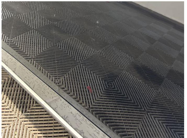
6: Door nsf Chipped 1 To 5
