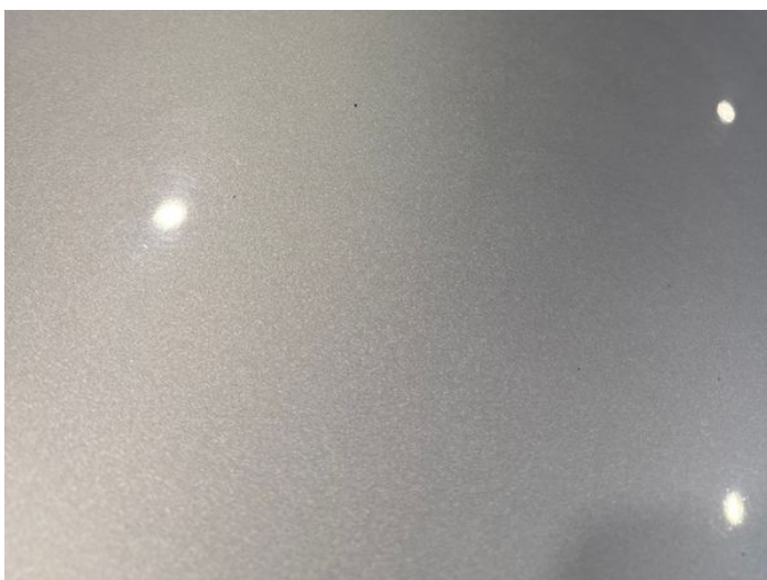
20: Roof Chipped 1 To 5
