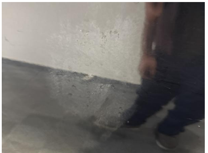
8: Door nsr Poor Previous Repair Poor Paint
