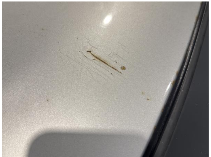
12: Roof Rusted Over 5mm
