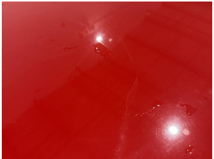
16: Roof Scratched Over 25mm Thru Paint
