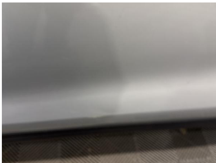
6: Door nsf Dented With Paint Damage
