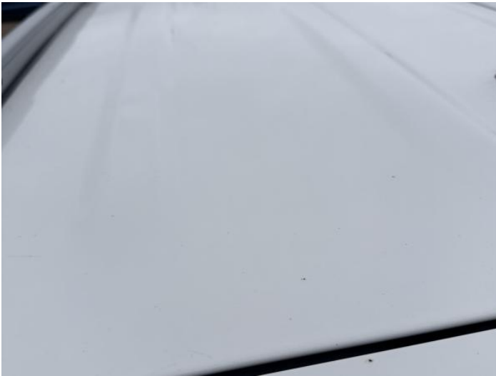
11: Roof Dented Over 30mm
