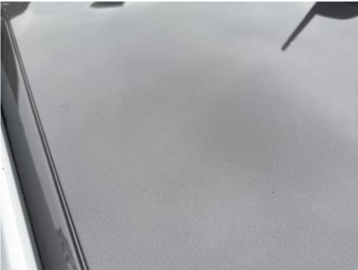
18: Roof Dented Between 10mm + 30mm
