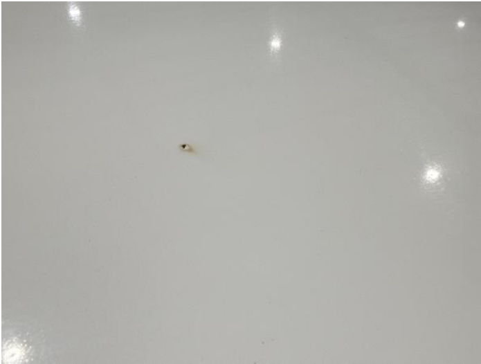
15: Roof Chipped 1 To 5
