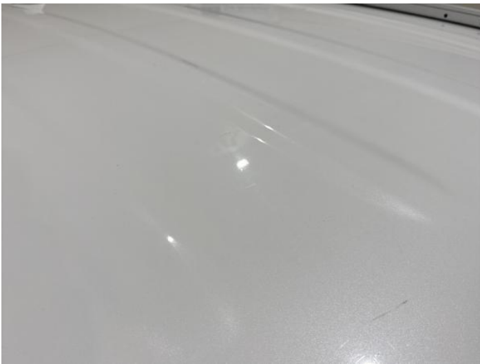
17: Roof Dented Over 30mm
