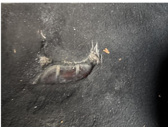
13: Carpets Front Torn Over 10mm
