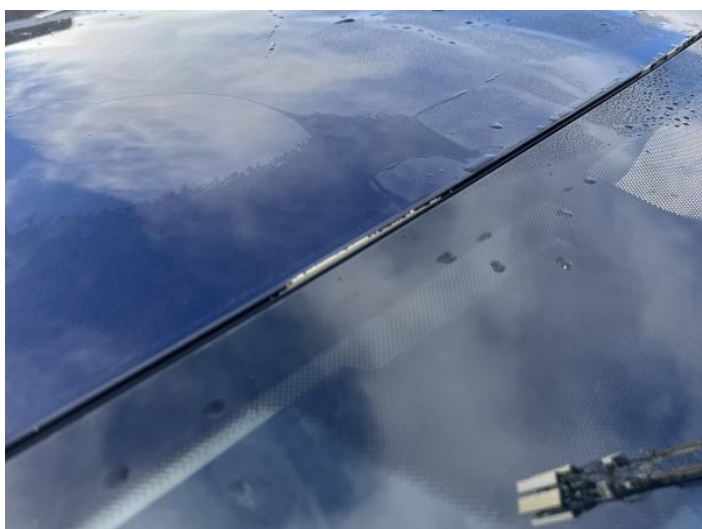
11: Roof Chipped Edge Chip
