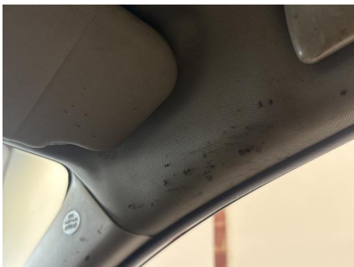
1: Roof Lining Burn UpTo 3mm
