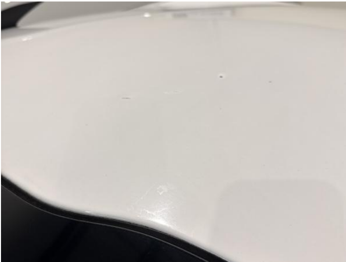
11: Roof Dented With Paint Damage
