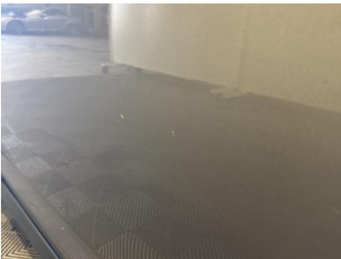
7: Door nsf Chipped 1 To 5
