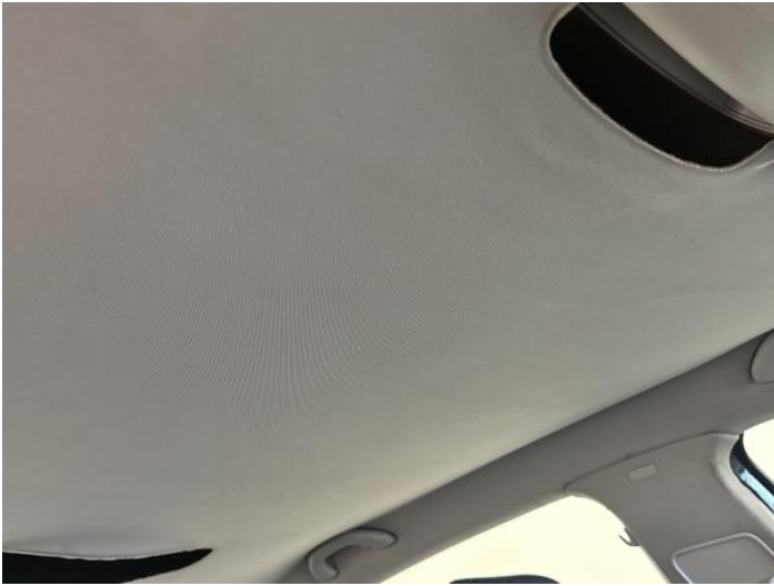
21: Roof Lining Scuffed Over 25mm
