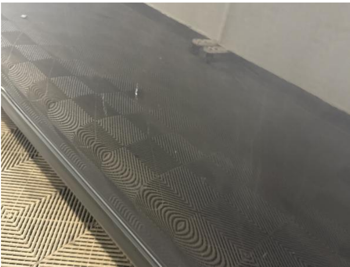
5: Door nsf Scratched Over 25mm Thru Paint
