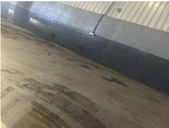
1: Door osr Scratched Over 25mm Not Thru Paint
