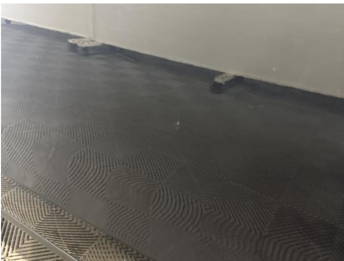
7: Door nsr Scratched UpTo 25mm Thru Paint
