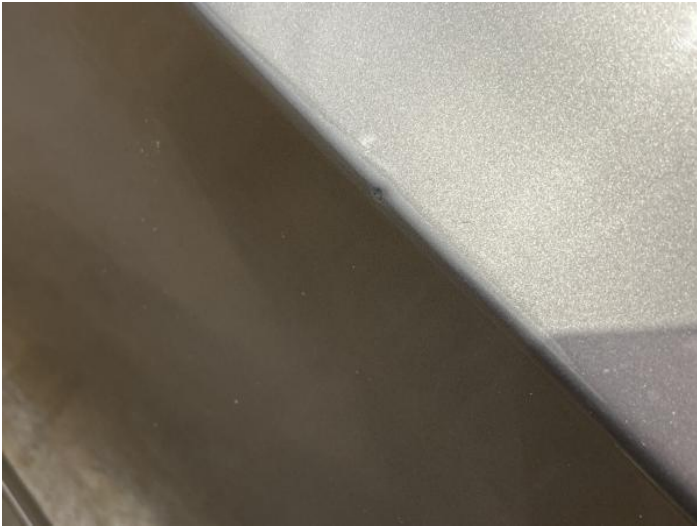
3: Door osf Chipped 1 To 5
