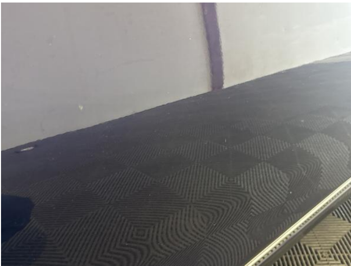
11: Door osf Chipped Multiple Chips
