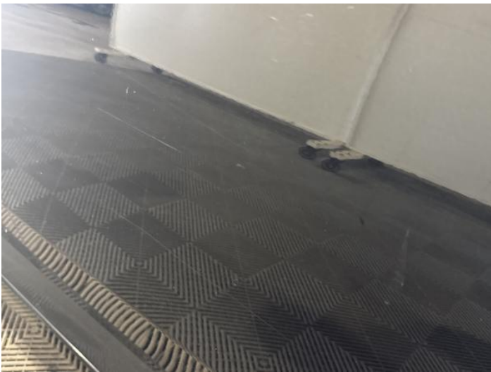
5: Door nsf Scratched Over 25mm Thru Paint
