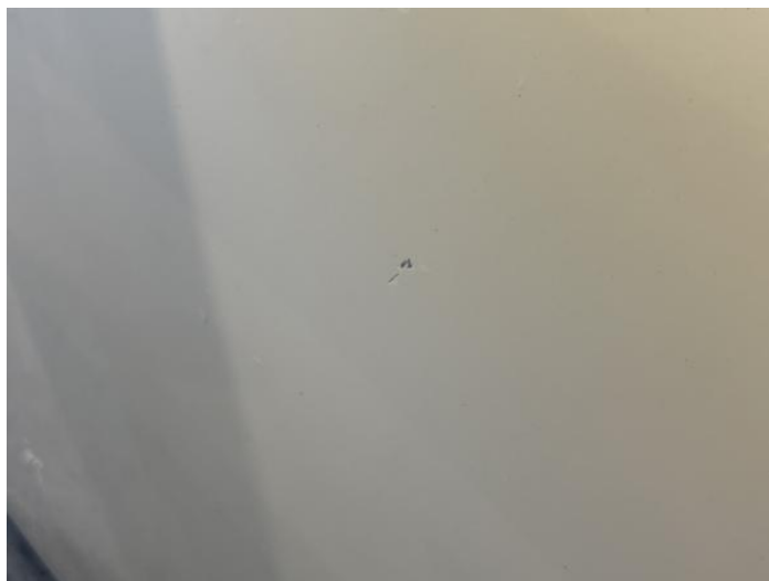
10: Door nsf Chipped 1 To 5
