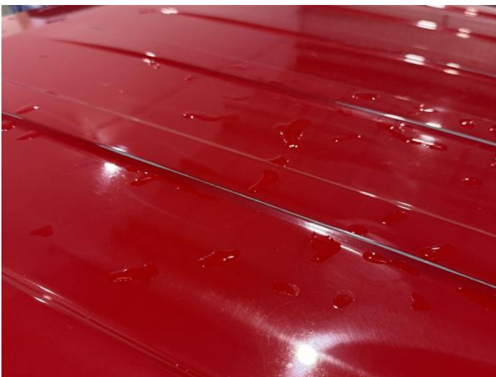
13: Roof Scratched Over 25mm Thru Paint
