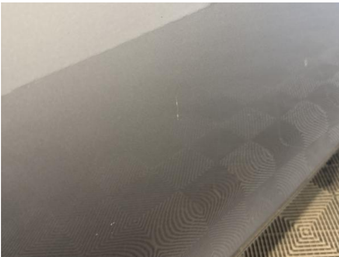
11: Door osf Scratched UpTo 25mm Thru Paint
