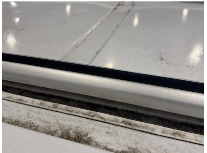
12: Roof Dented Over 30mm
